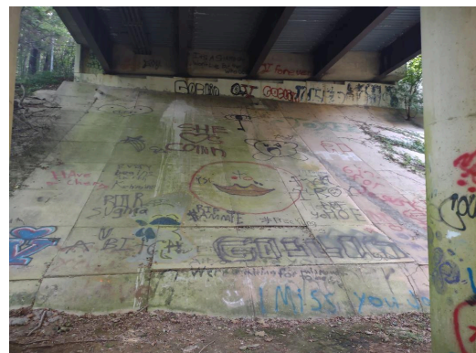
Graffiti, Great Seneca HWY bridge. By Mike Calabrese
